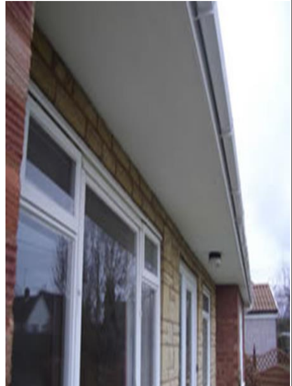
Pieces of Asbestos Insulating Board (AIB)
